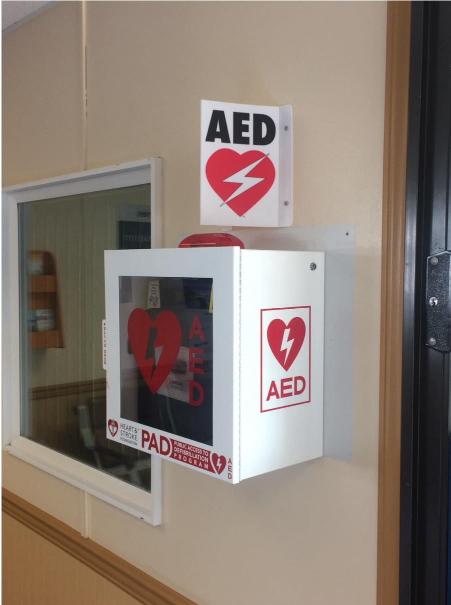
The new AED installed in the waiting room at Long Harbour terminal.
